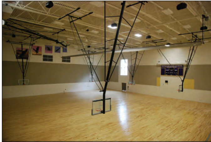
Main gym, basketball backboards/hoops in place. Wood floor completed with first coat of finish. Scoreboards and eagle graphics relocated from original gym.
