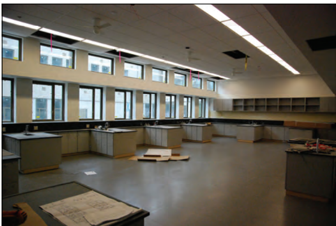
Science lab nearing completion. Ceiling tiles, fans, lights installed and flooring complete.
